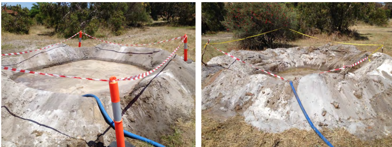
Figure H1: Infiltration Testing at Bayswater Dive Structure (Pit 1 left, Pit 2 right)
