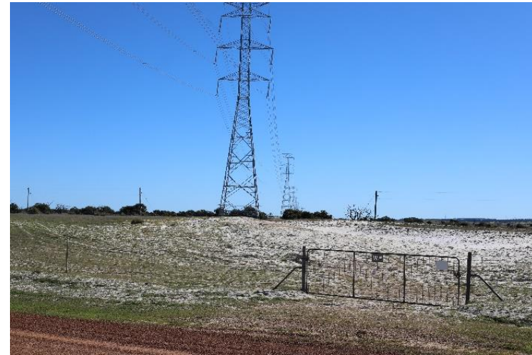
Figure 8-1 Transmission line traversing rural property at Hunter Road, Regans Ford. Towers are at approximate 550m intervals, with the first one approximately 400m in the distance and the second approximately 950m in the distance (image: Aurecon, August 2025)
