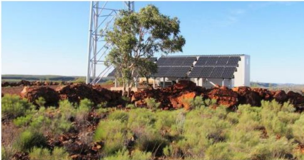
Communications equipment on Nate Hill may require particular attention during bushfire to prevent damage to solar panels.
