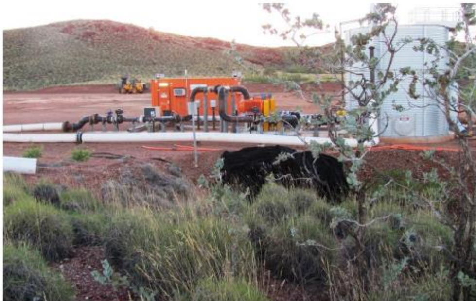
The return water pump facility is located close to flammable vegetation.
