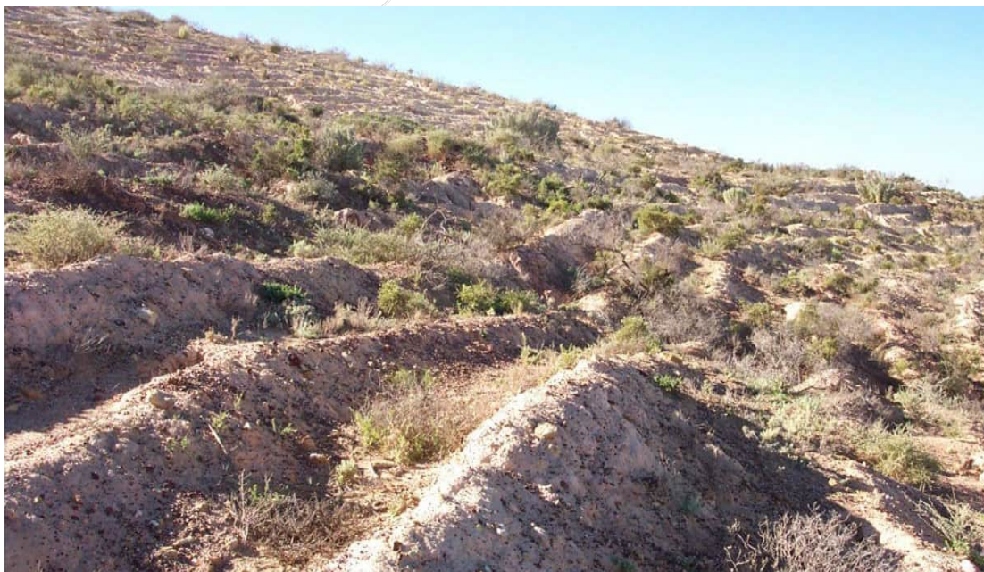
Figure 8: Example of a laterally irregular batter slope shapes. Irregularity caused by poor construction and was not part of the rehabilitation design.
