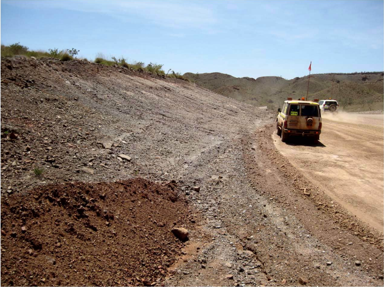
18. Cut shale on North road side
