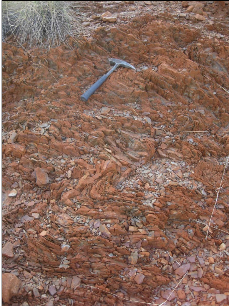
PHOTOGRAPH 2 - FOLDED SHALE AT TSF EMBANKMENT
