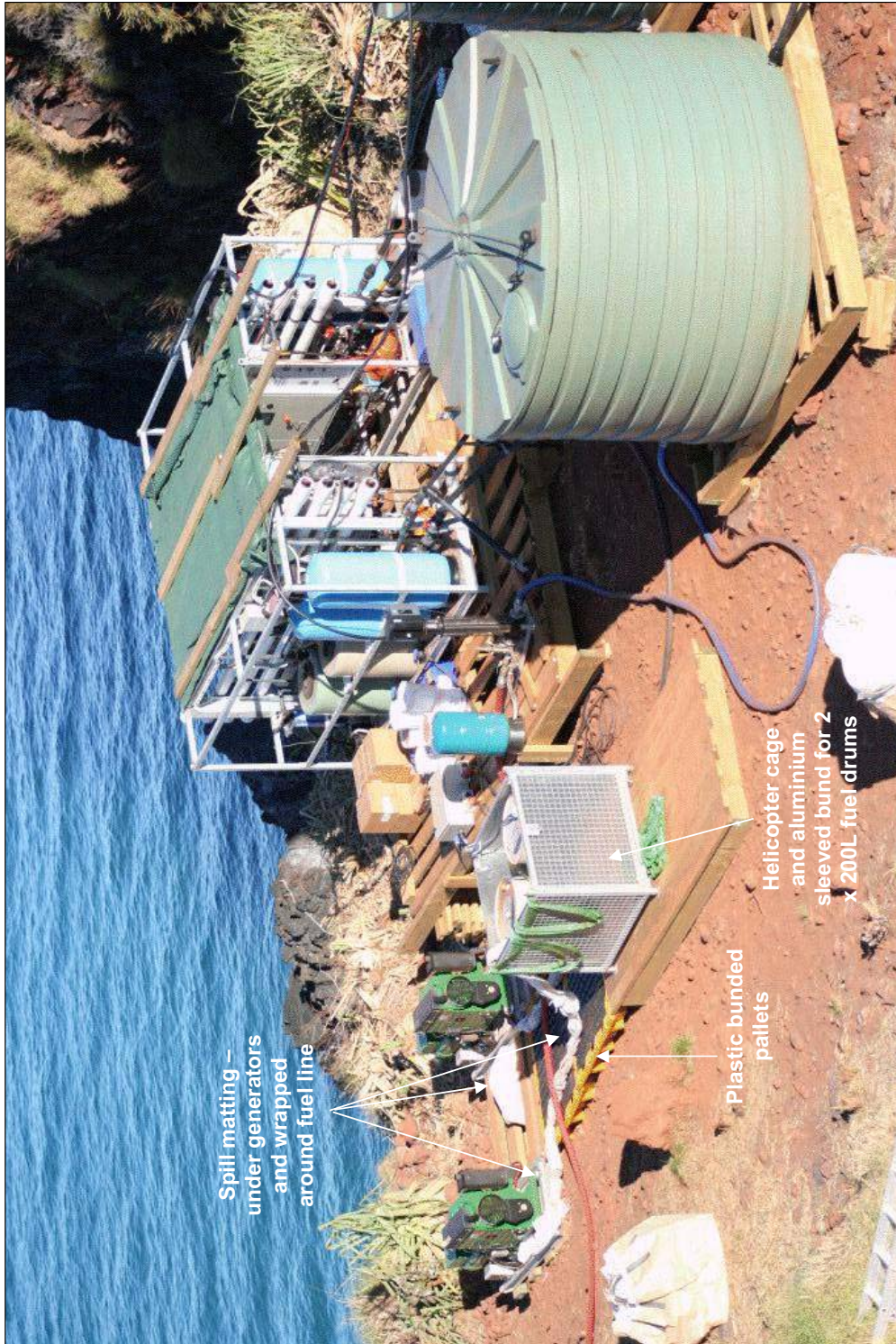
Plate 6 Desalination plant at Hardstaff peninsula and deep water inlet/outlet point
