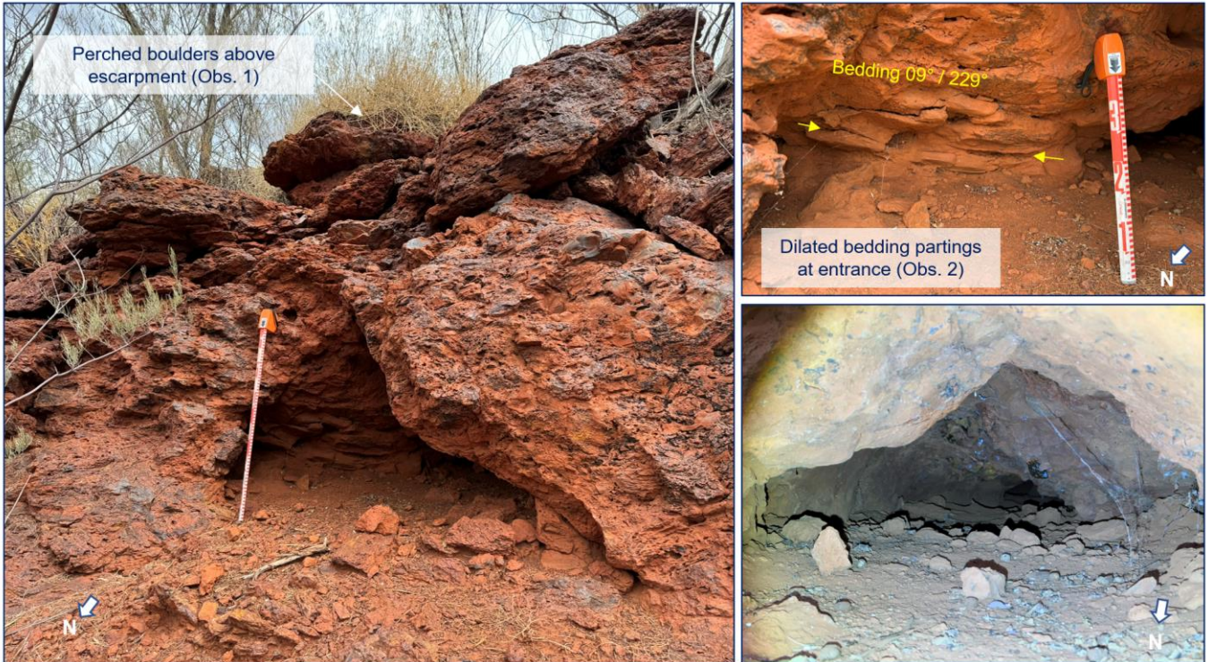
Inset 18: Engineering geological observations of cave MEC072. Left: Cave entrance viewed towards the southeast showing perched boulders above the escarpment. Top Right: Bedding partings observed inside the cave entrance. Bottom Right: Cave interior viewed towards the south.
