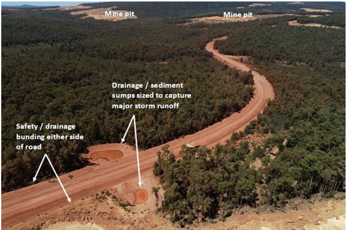
Plate 2-8 Myara Mine haul road drainage
