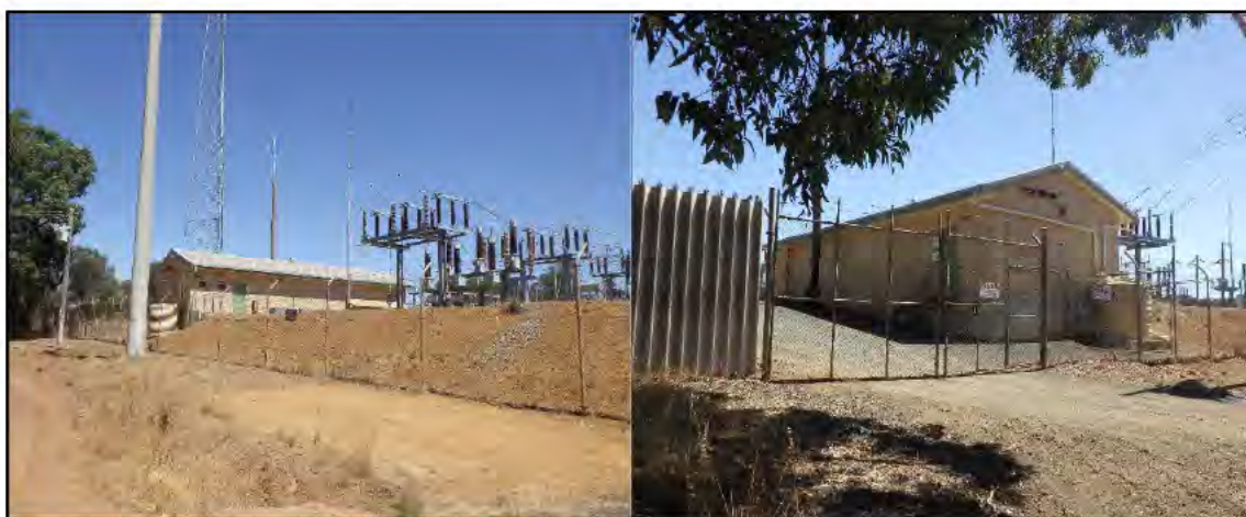
Figure 17: Views of the Western Power Kojonup Sub Station on Tunney Road.
